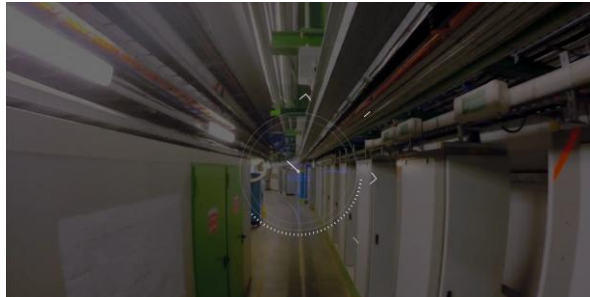
Train Inspection Monorail
